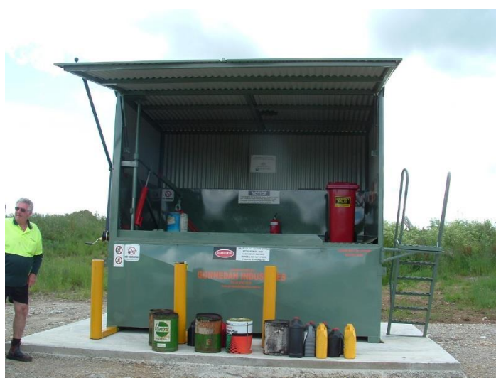
Figure 22 Waste Oil Collection Unit
